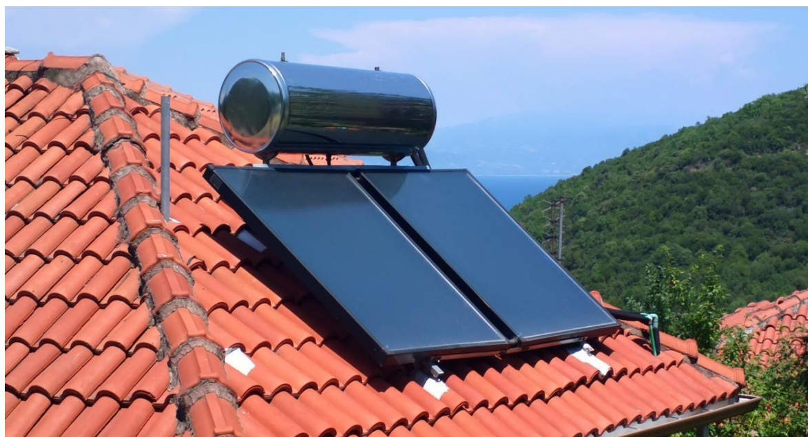
Image 9 - Solar thermal energy installation ©Adobe Stock, Springtime78
